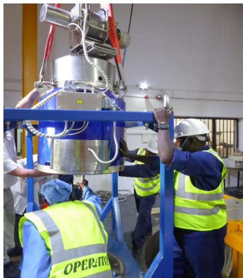
Transfer cask installation
