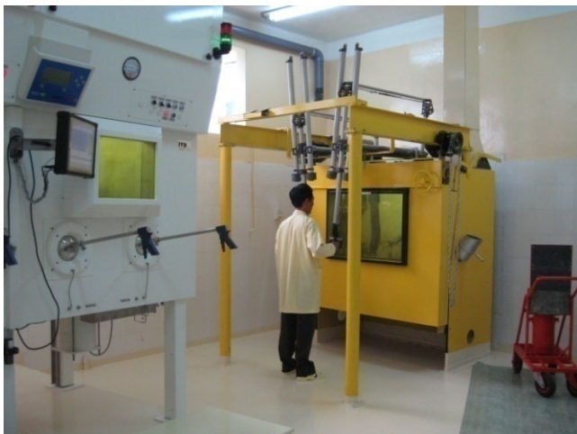
Hot cell and I-131 production line
