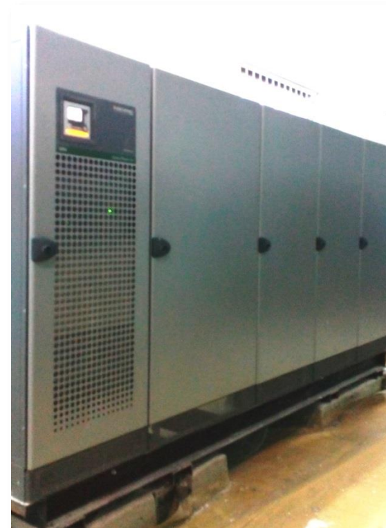
Batteries 30 KW, 6 hours
