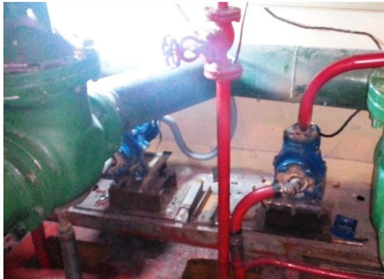
2 pumps, 45 m 3 /h each instead of 10 m 3 /h for HEU core
