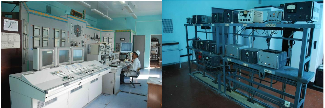
Pic. 4 Old and new CPS installed and operating in parallel
